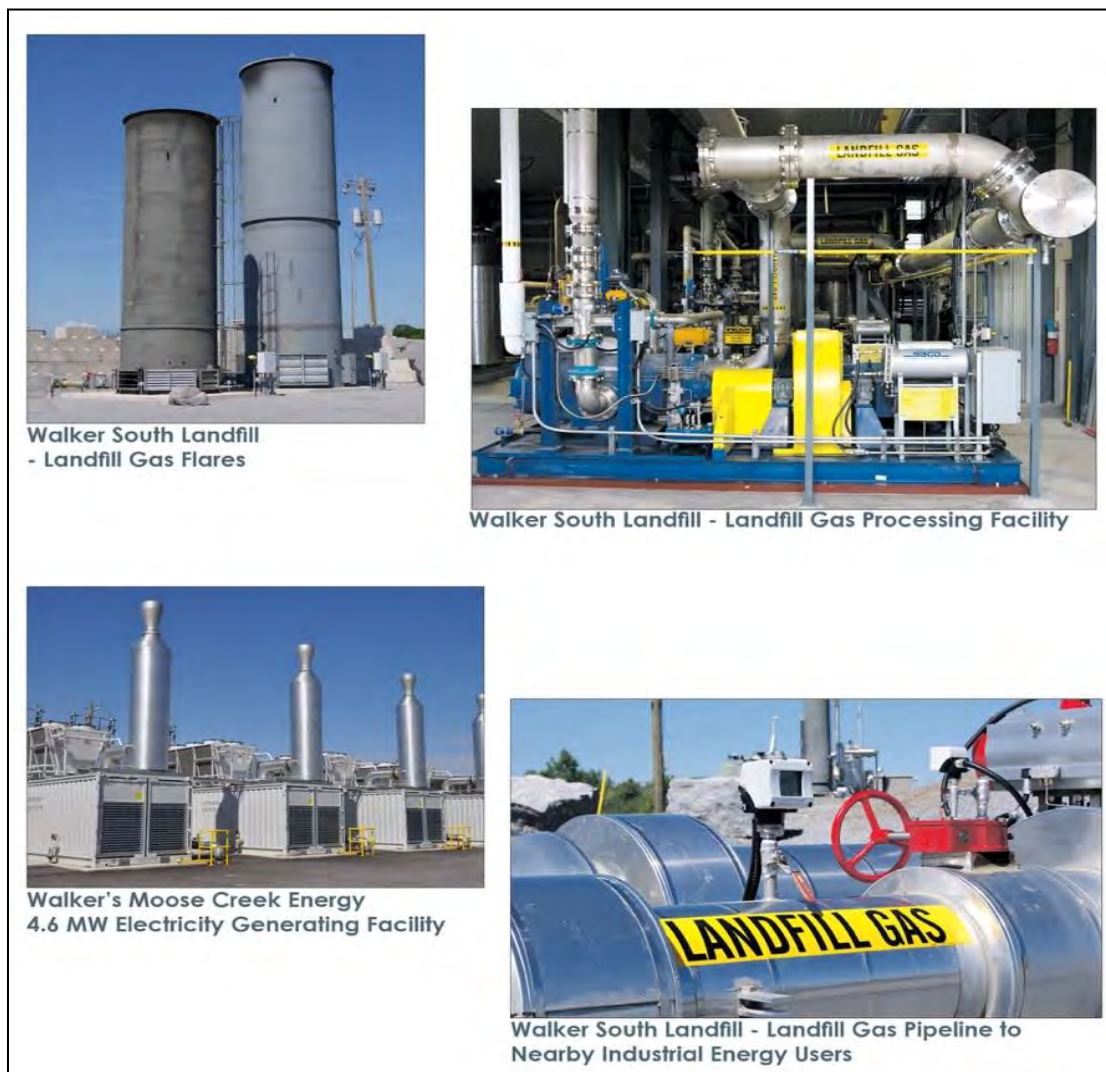
Figure 6-10: Examples of Landfill Gas Management Facilities
