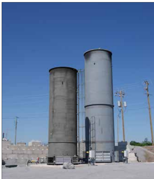
Walker South Landfill - Landfill Gas Flares
