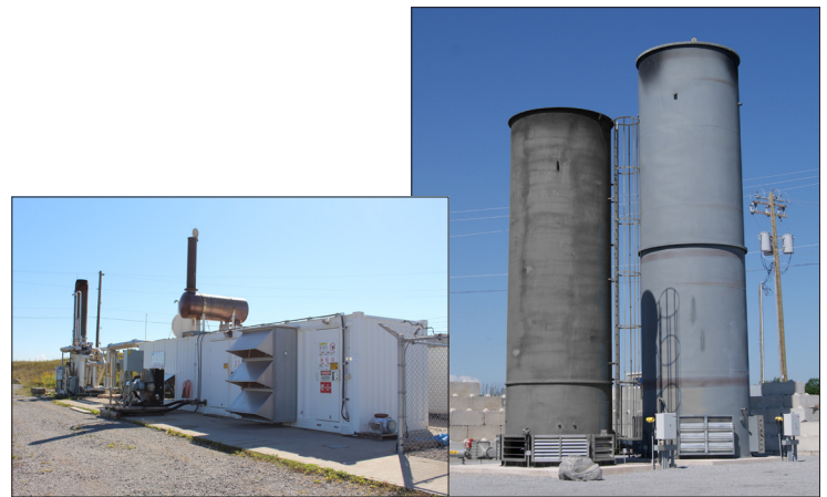
Walker South Landfill - Landfill Gas Flaring & Utilization Facilities
