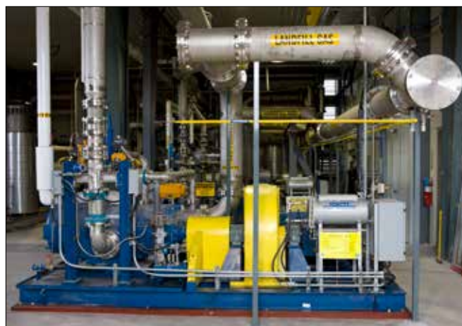
Walker South Landfill - Landfill Gas utilization infrastructure.
