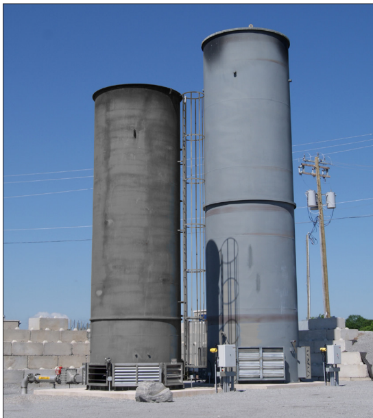
Walker South Landfill - Landfill Gas Flares
