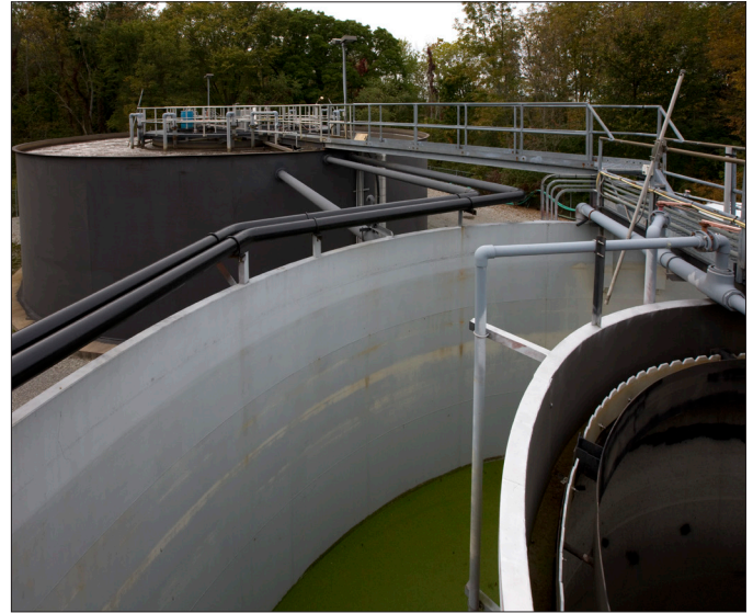
An Example of a Leachate/ Wastewater Treatment Plant
