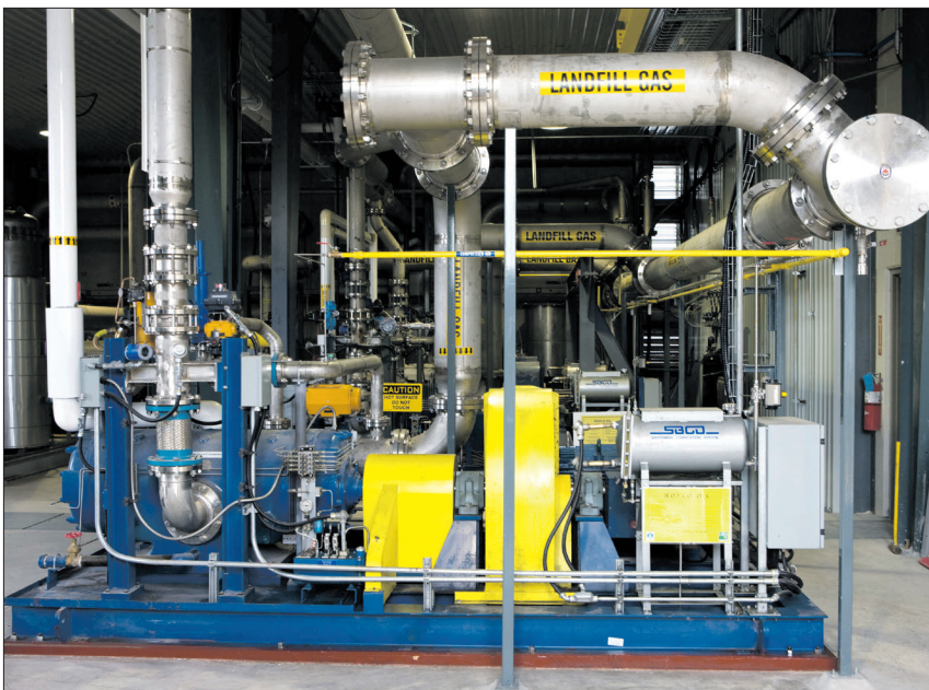
Walker South Landfill - Landfill Gas Processing Facility
