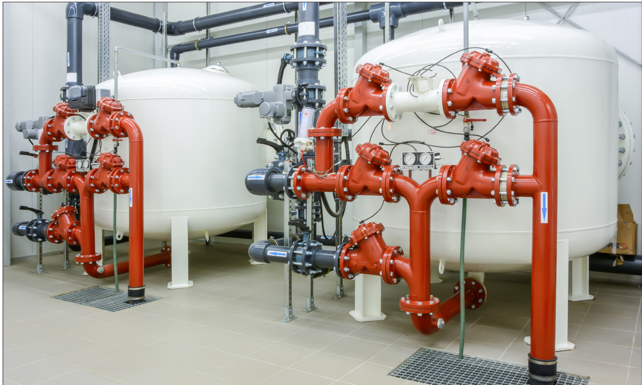
Example of Typical Leachate Treatment Equipment
