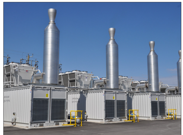
Walker's Moose Creek Energy 4.6 MW Electricity Generating Facility
