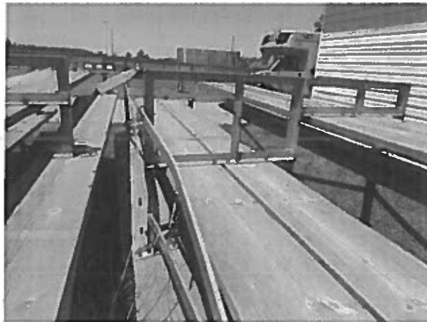
BENT AND DETACHED CROSS BRACING
