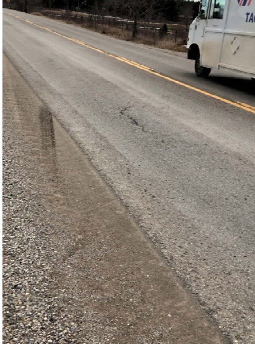
Exhibit 9-11: Highway 401 Longitudinal Cracking
