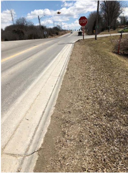
Exhibit 9-9: County Road 6 and Beachville Road Northbound Rutting
