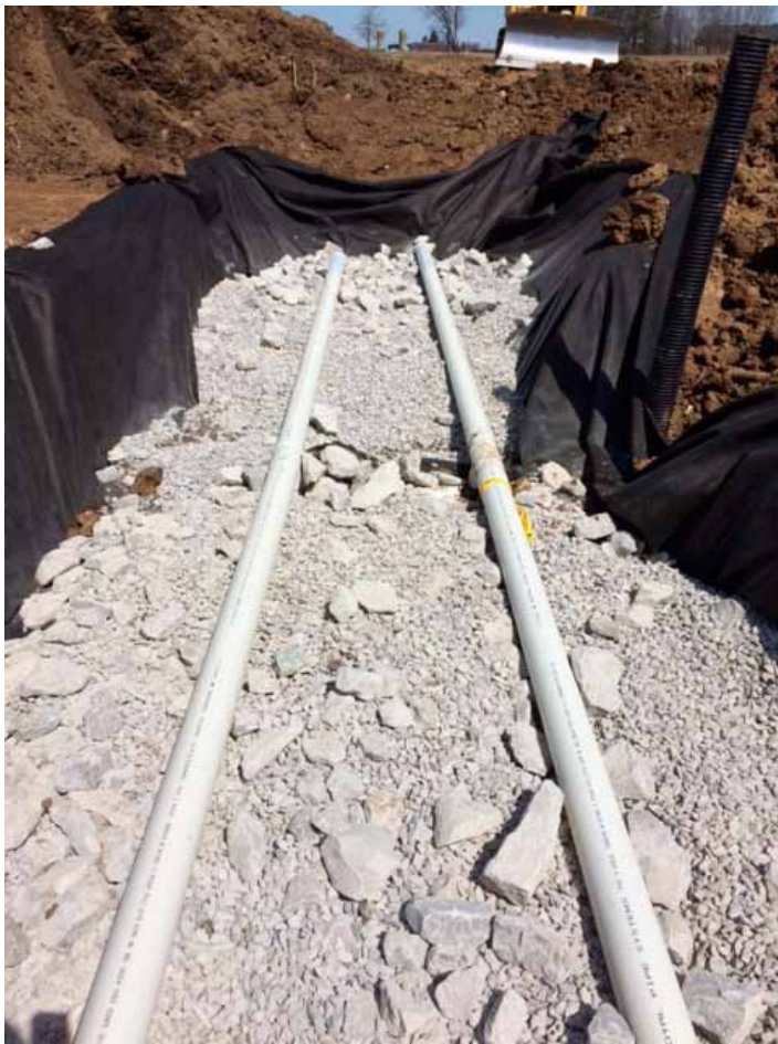
The blind inlet is a series of perforated plastic pipes surrounded by gravel and wrapped in filter cloth. The black pipes will provide access for water quality and quantity monitoring.
