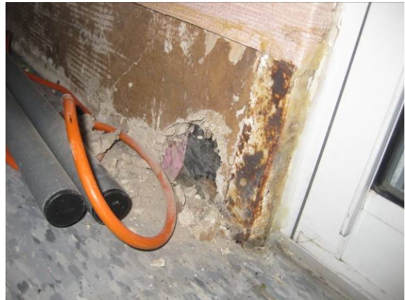
Photo 8 - Mech'l room (before)
