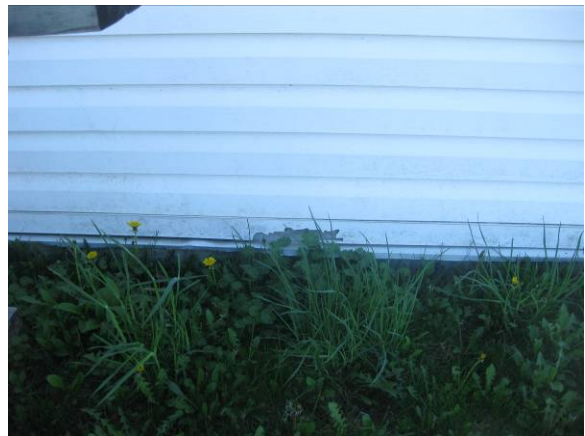
Photo 18 - Holes in siding
