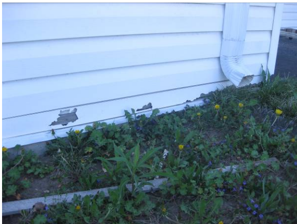
Photo 21 - Short downspout, rotted siding
