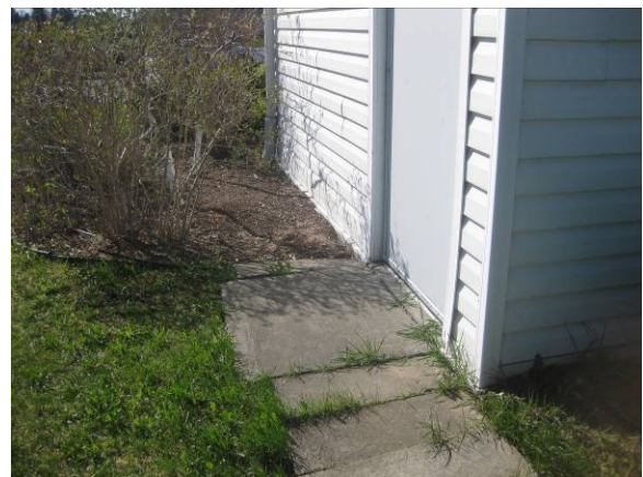
Photo 24 - High exterior grade at building
