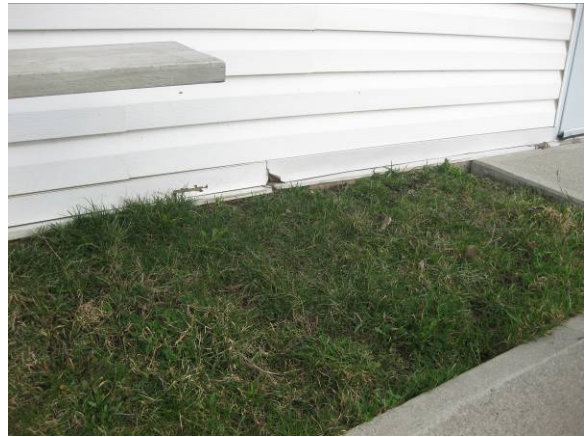
Photo 16 - Base of siding in poor condition
