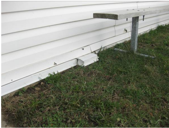
Photo 15 - Holes in siding
