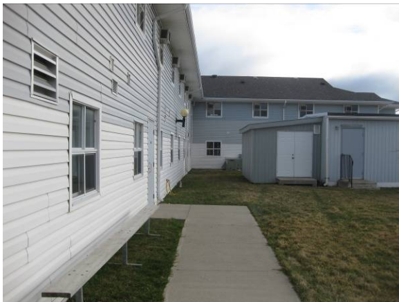
Photo 17 - High exterior grade at building
