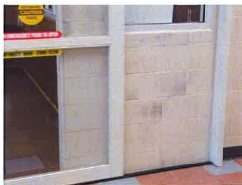
Figure 13 – Painted block requires painting
