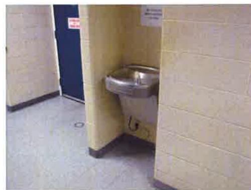
Figure 14 – Drinking fountain is not considered accessible
