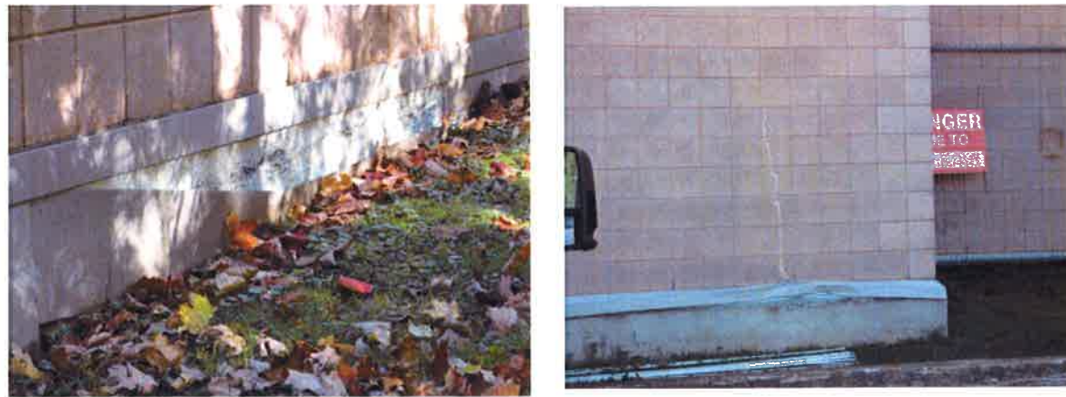
Fig. 7 – parging is damaged and requires repair
